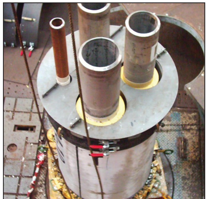
ZERON 100 Pipe riser used in an offshore oil platform riser.
